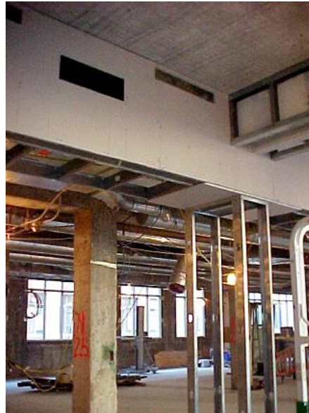
Figure 37 - Bulkhead Housing FPIUs (2)
